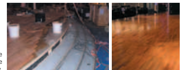
Installing the hardwood onto the support layer for the Crystal Cruise Line's ship, Crystal Serenity.
