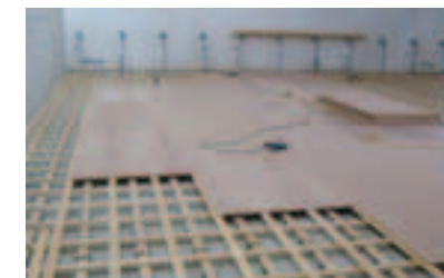
Photos show installation of Harlequin WoodSpring at Scottish Ballet studios, Tramway, Glasgow
